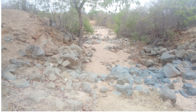
Figure 6: Sanga river dam wall (broken)
